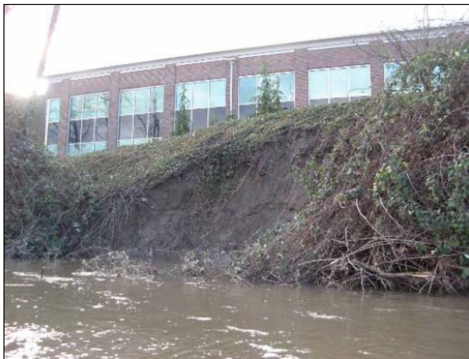
Figure 4-2. Slope erosion and slumping failure – Lower Green River (King County, 2006)
