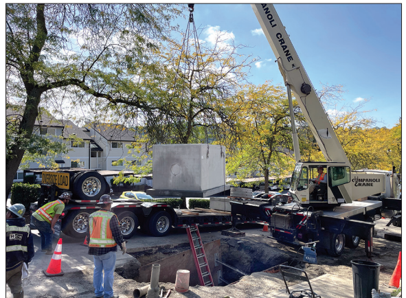
Installed a 14-Ton water vault due to the difference in water zones
