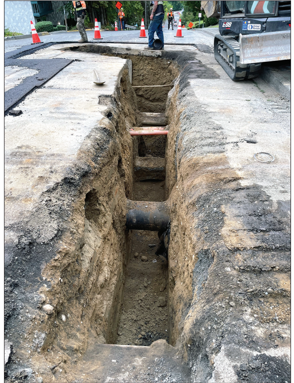
Intersection of 152nd and 57th presented numerous utilities to avoid, including fiber, gas, high voltage lines, and a large water main
